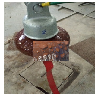
Figure 17: Test cement dust pollution, HC=4.
