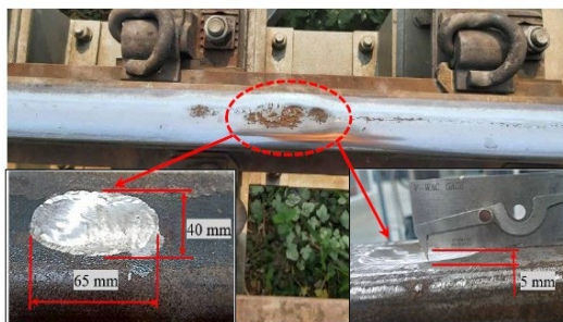
Figure 3: Surface wear groove on an in-service R260 grade.
