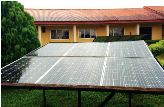
Figure 2: Array of Solar Panels where data was captured.
